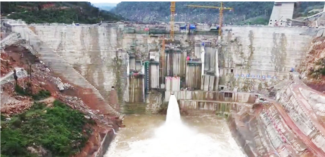
Construction of the project started in 2017, the reservoir impounding began in June 2021 and commissioning is scheduled for mid 2022.
